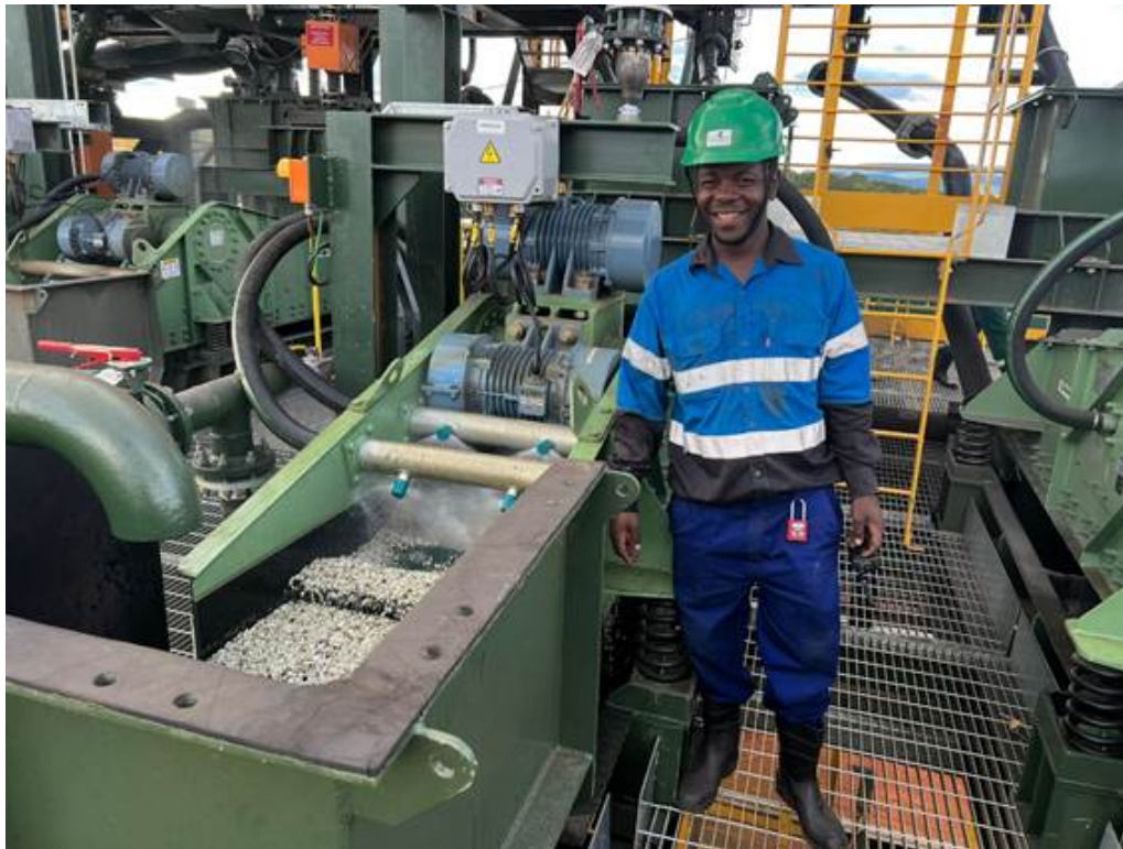
Figure 1: Completion of DMS Commissioning and First Production of Green Lithium
